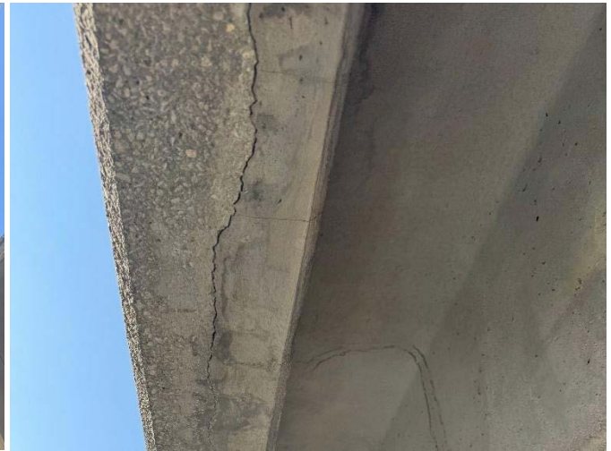
Spandrel Crack at East End of Structure
