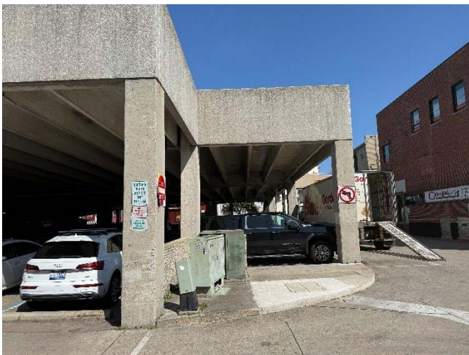
Southeastern Column with Vehicular Damage
