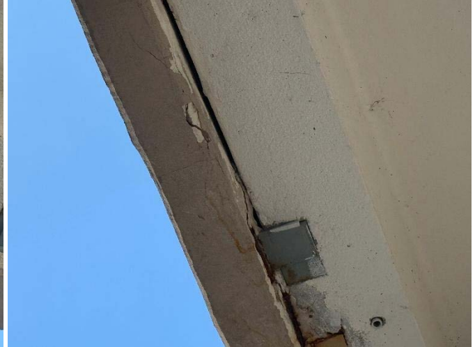
Cracks in Pedestrian Bridge Spandrel Panel
