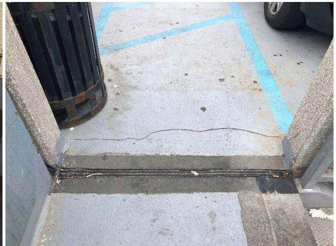
Crack Between Pedestrian Bridge and Structure
