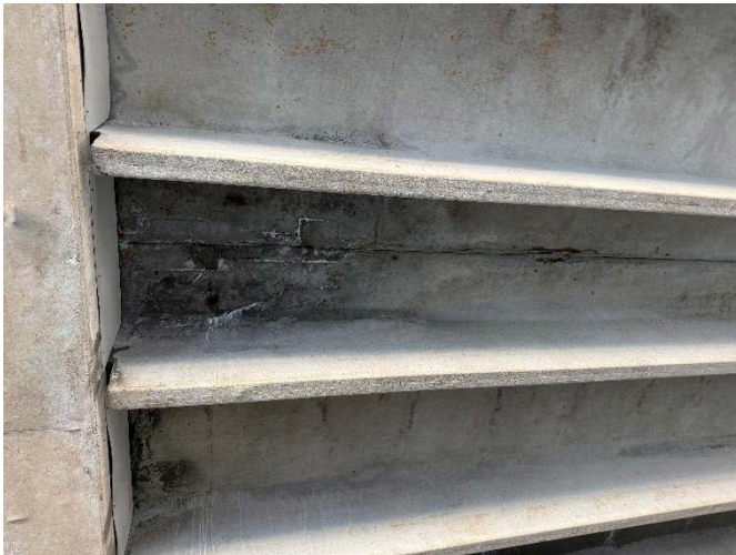
Degradation of Tee Flanges
