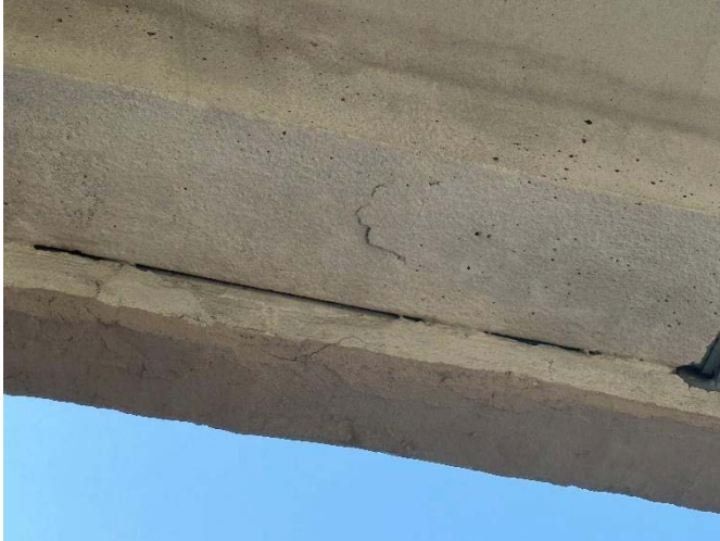
Cracks in Pedestrian Bridge Spandrel Panel
