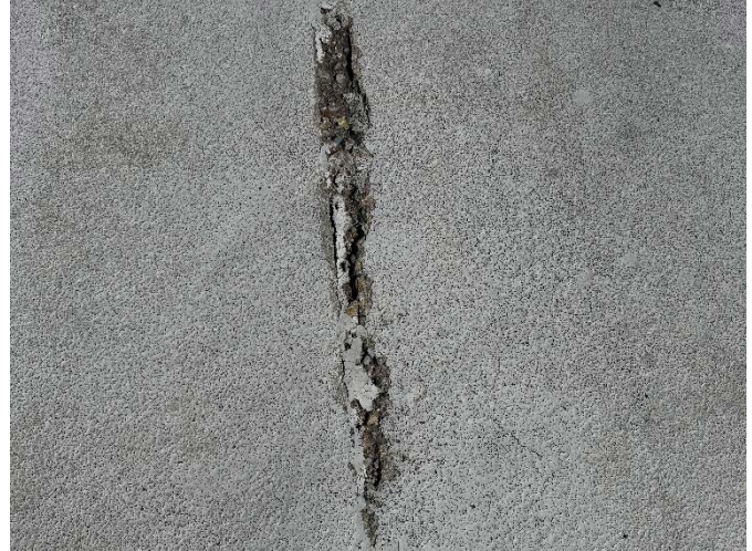
Area of Deteriorated Traffic Coating and Concrete
