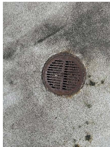
Debris in Drain
