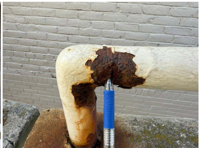
Hole in Handrail
