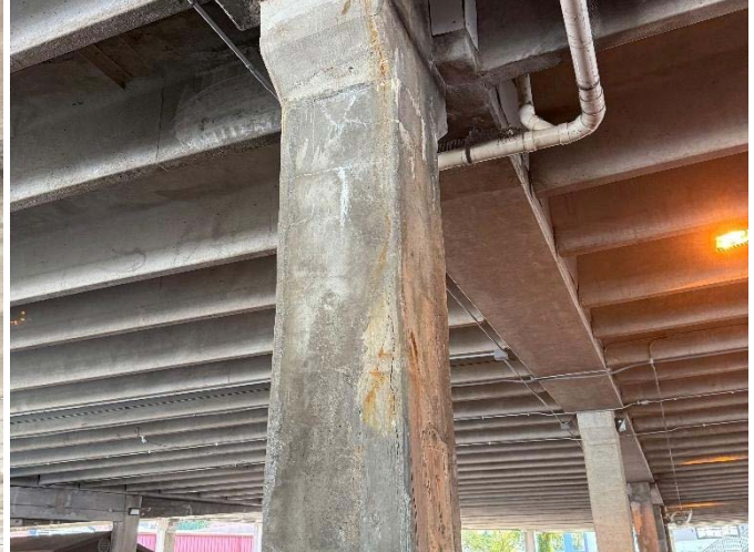
Concrete Cracking at Column
