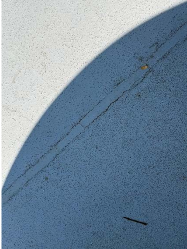
Failed Joint Sealant
